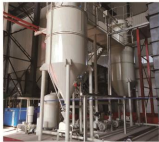
低压输送系统 Low pressure conveying system
