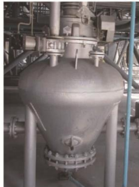
高压仓泵输送系统 High pressure transport conveying system
